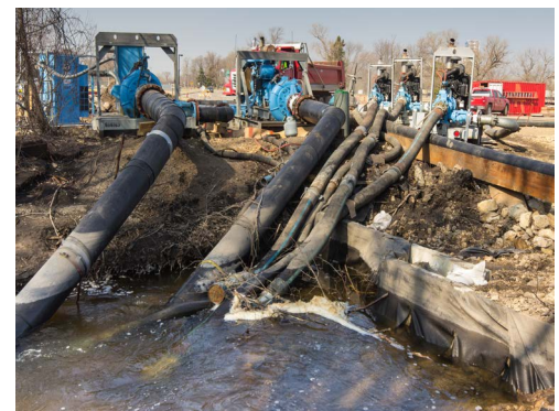
Figure 6. Drain all water from equipment where water may be trapped. Remove drain plugs and drain hoses prior to transport. Photo Credit: Peter Leete, DNR
