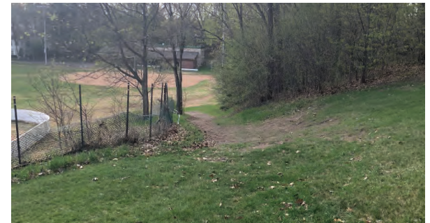
Existing hillside showing erosion on non-accessible route.
